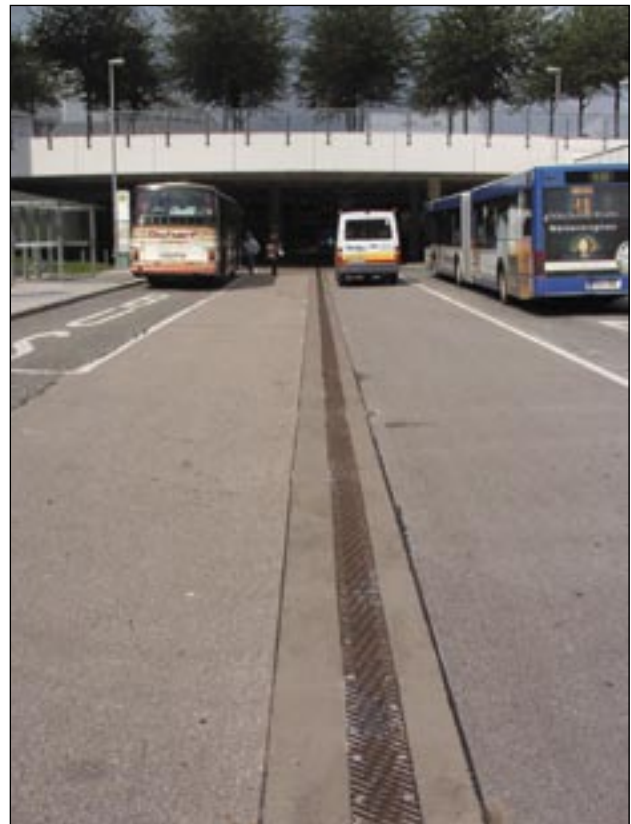
South bus station of the "Franz-Josef Strauss" airport, Munich: Repairing drainage channels
